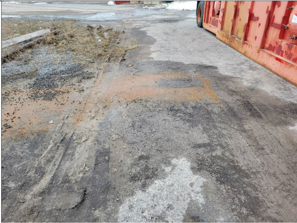
Photograph 3 (March 27, 2023). Evidence of leakage following tank removal.
