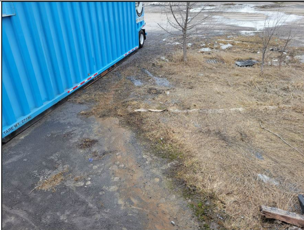
Photograph 5 (March 27, 2023). Evidence of leakage following tank removal.
