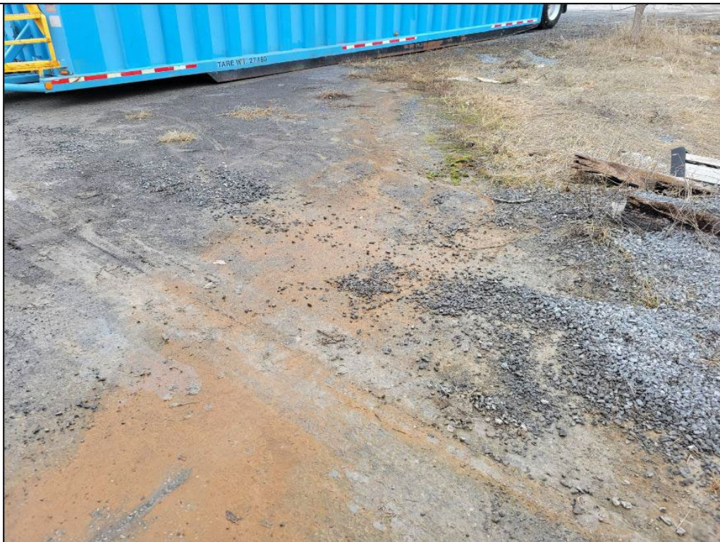
Photograph 4 (March 27, 2023). Evidence of leakage following tank removal.
