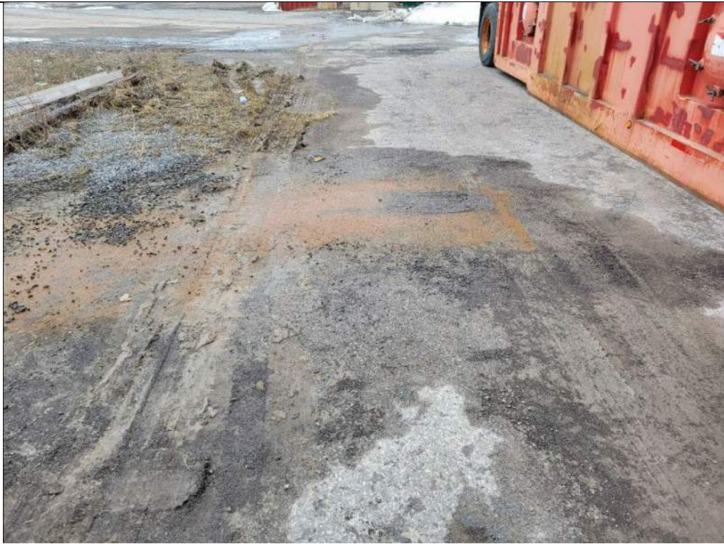
Photograph 3 (March 27, 2023). Evidence of leakage following tank removal.
