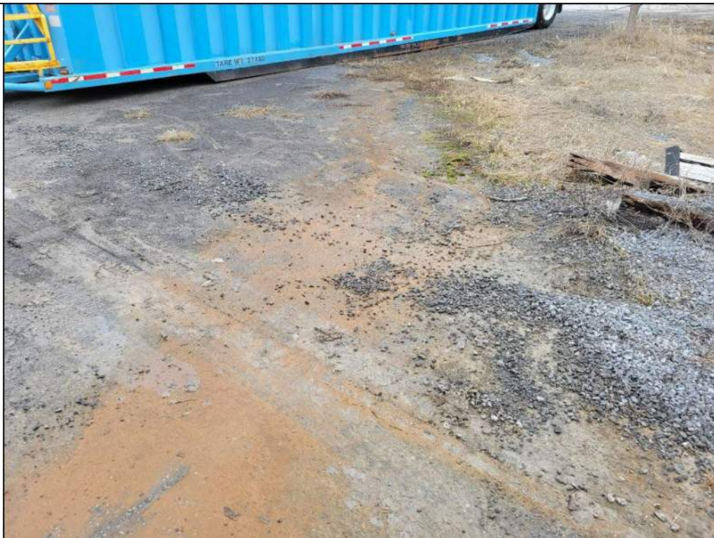
Photograph 4 (March 27, 2023). Evidence of leakage following tank removal.
