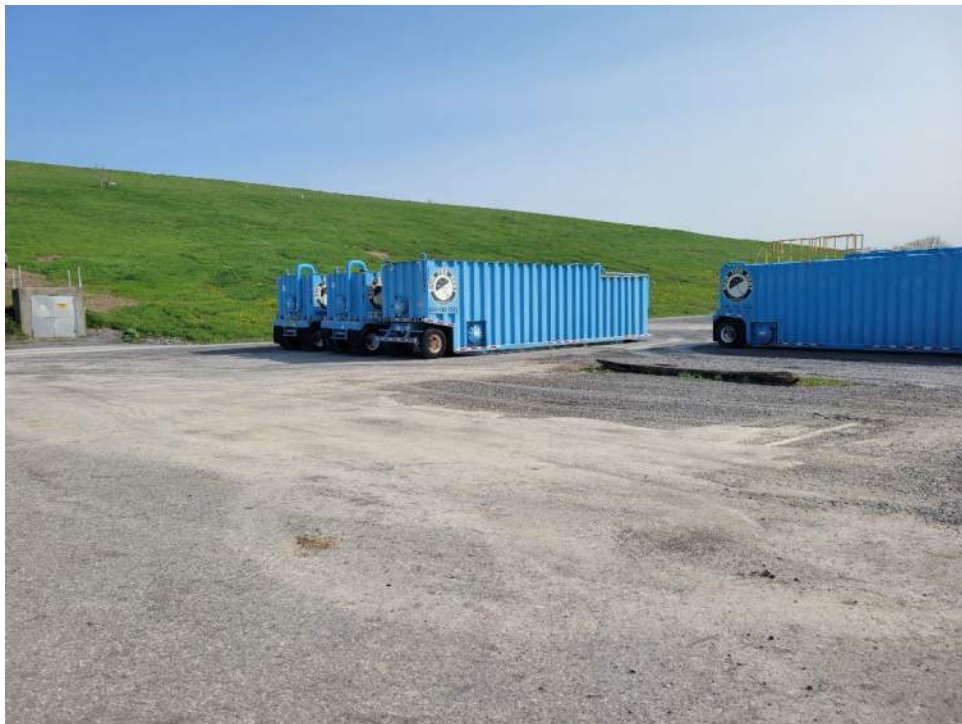
Photo 4: Site conditions following removal of impacted soil and final grading with clean gravel (May 8, 2023)
