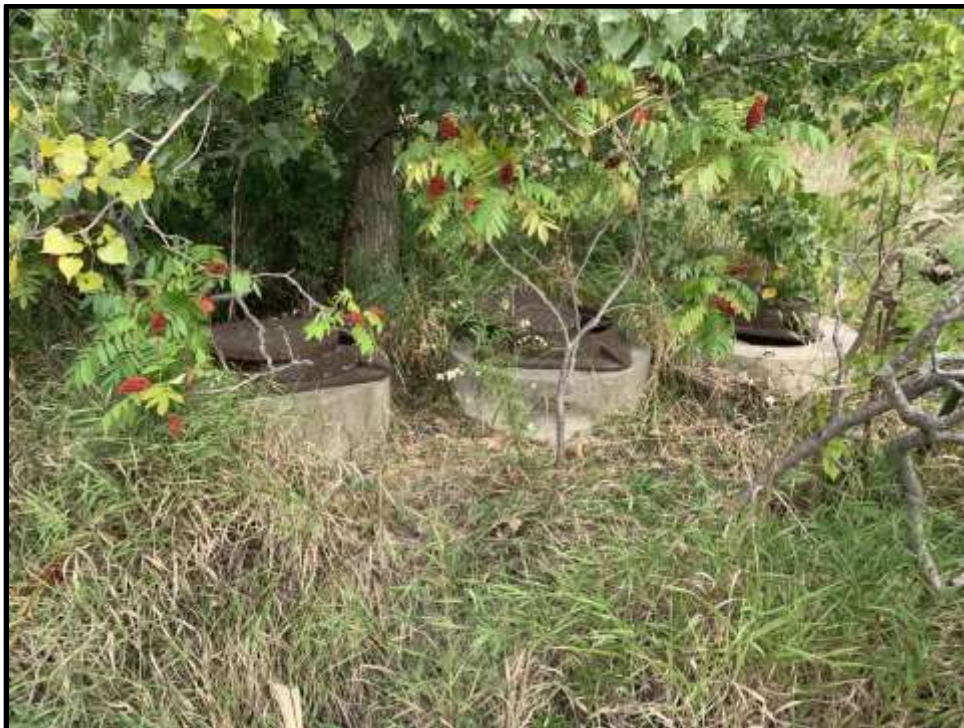
Photo 42: View of the dislodged lids south of the former contaminated soil pad. No "Confined Space" signage is present.
