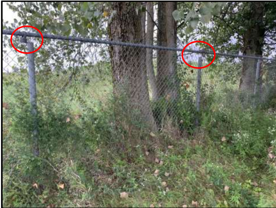
Photo 2: View facing southeast of the chain link fence along the east side of the landfill entrance. The posts have separated from the top rail.
