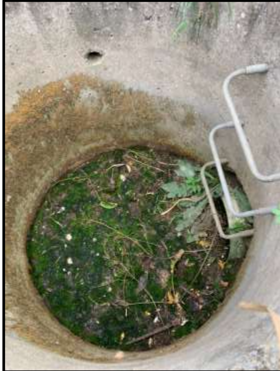
Photo 21: View inside drop inlet pipe structure at Stormwater Pond 2. Sediment is present in the structure but does not obstruct flow.
