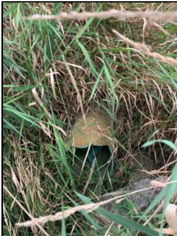
Photo 32: View of the outlet pipe from the drawdown structure at Stormwater Pond 1. No evidence of silt exiting the pond was observed.
