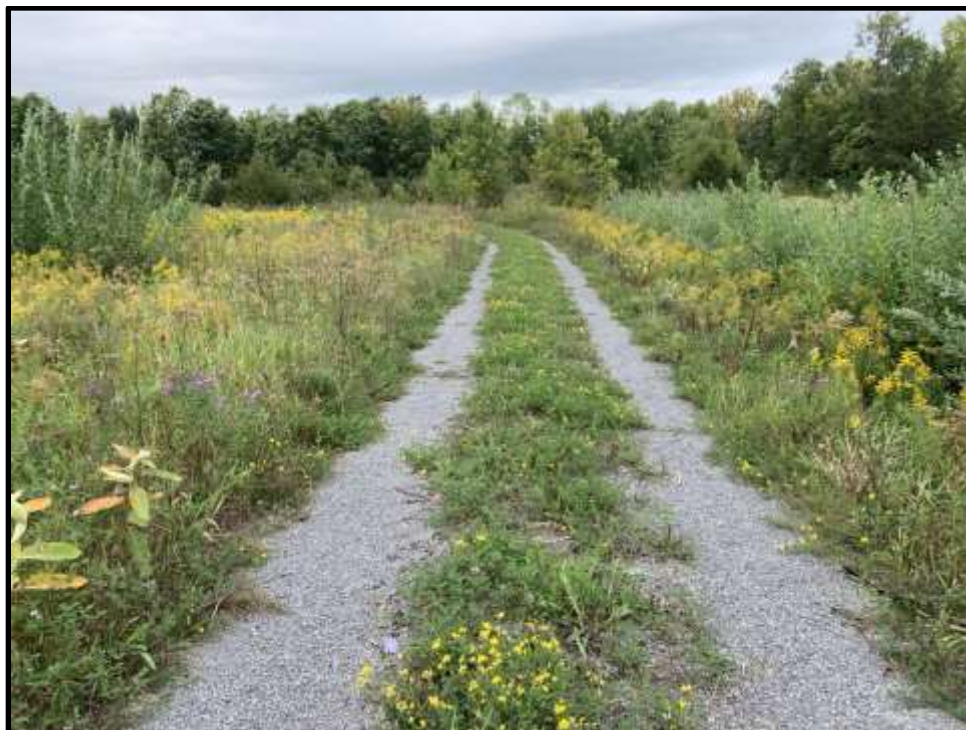
Photo 16: View facing north of the access path leading to Stormwater Pond 2. The path is in good condition.
