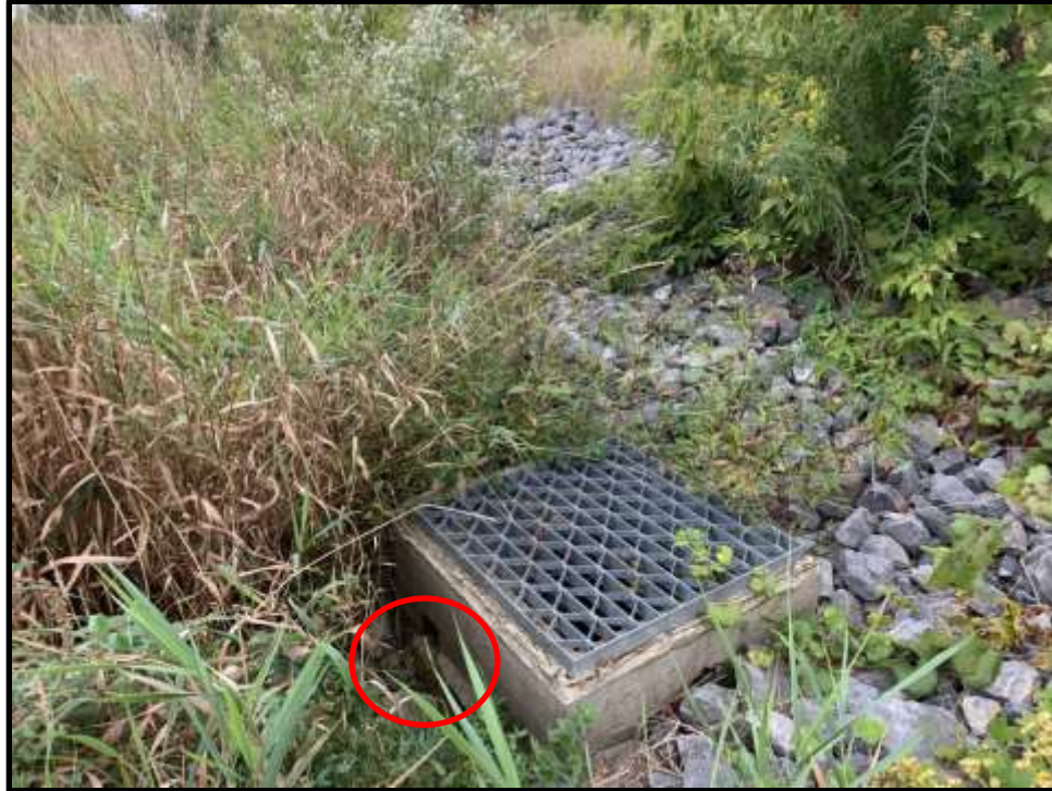
Photo 11: View facing southwest of the inlet structure at the west end of Stormwater Pond 3. The inlet to the structure (circled) is presently clear, but vegetation is beginning to encroach the area.
