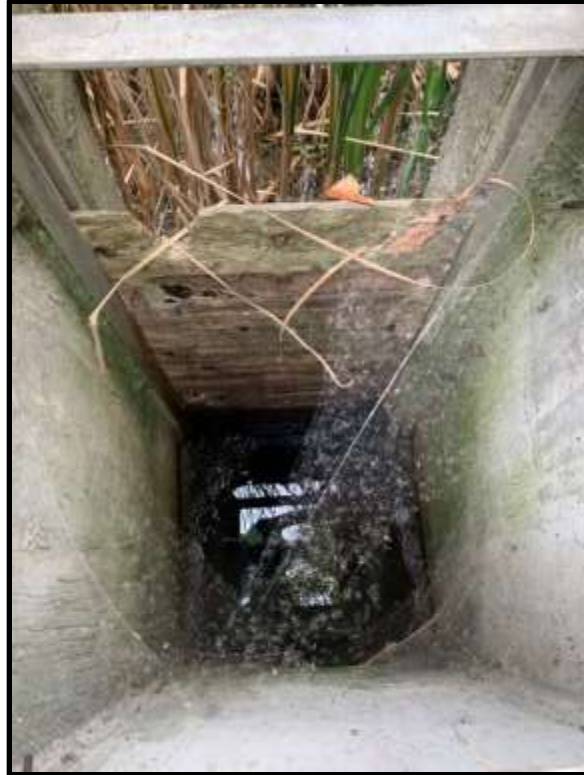
Photo 19: View of the stop logs present within the drawdown structure of Stormwater Pond 2.
