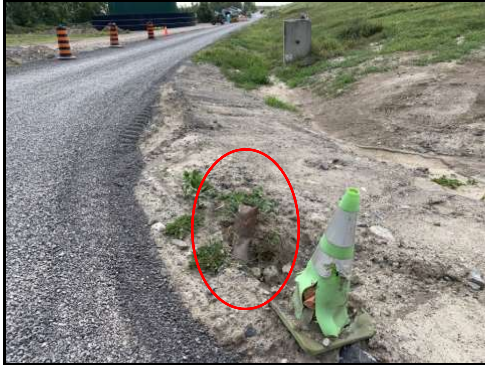
Photo 35: View (encircled) of monitoring well M19 on the southeast corner of the landfill. It is not clear if the well is part of the site's monitoring network.
