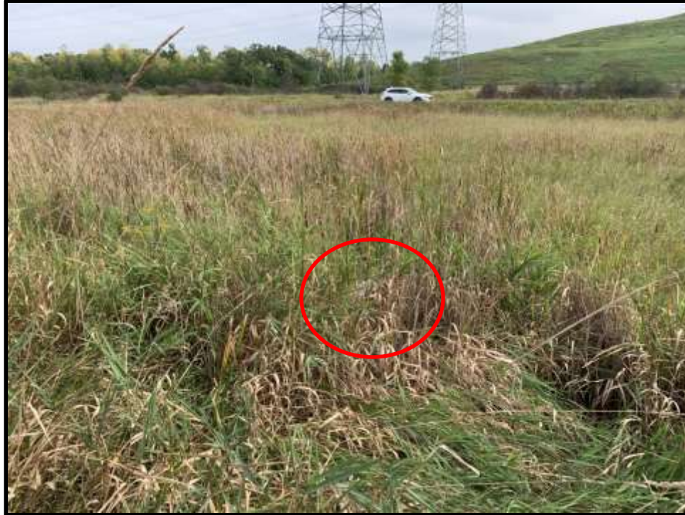
Photo 29: View of the drop inlet pipe structure (circled) at Stormwater Pond 1. Vegetation has obscured the structure.
