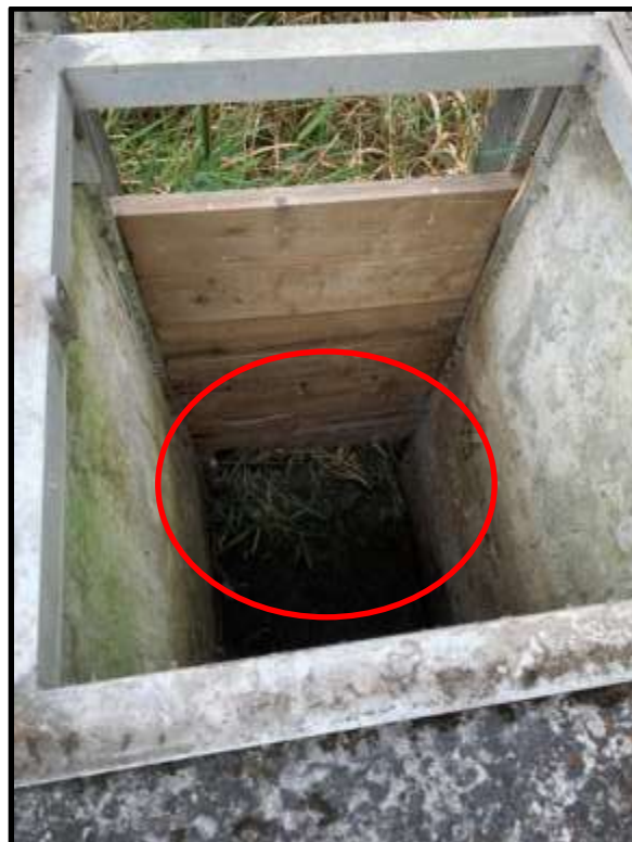
Photo 28: View of the stop logs inside the draw down structure at Stormwater Pond 1. Boards at the base of the structure have rotted and require replacement.
