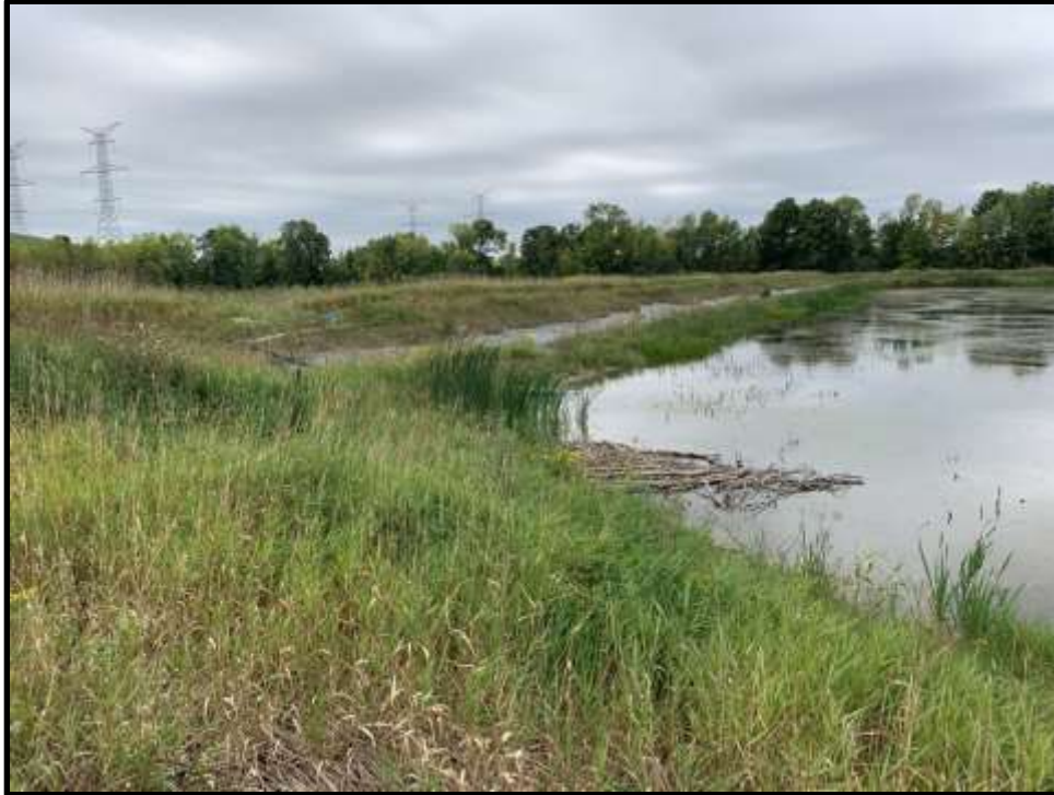
Photo 23: View facing southwest of the leachate holding lagoon. Debris shown in the water may be evidence of a former beaver dam. No evidence of rodents (no damage to the HDPE liner) was observed.
