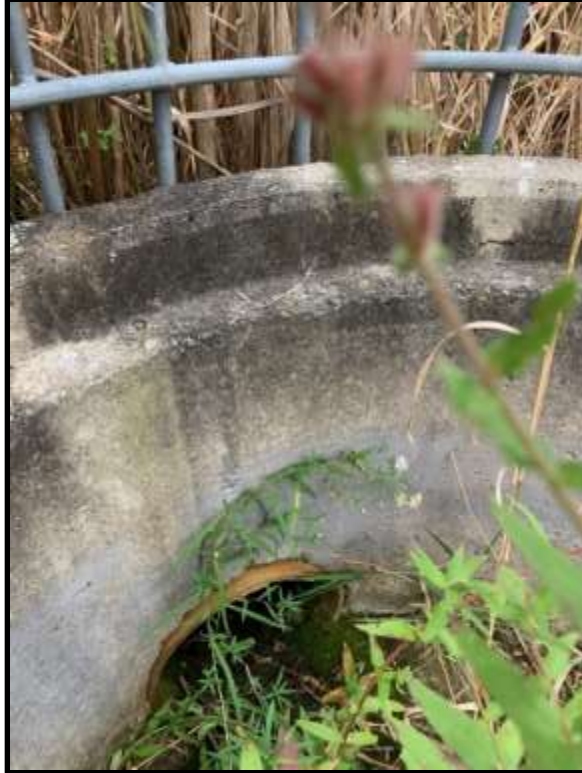
Photo 31: View of the inlet pipe of the drop inlet pipe structure at Stormwater Pond 1.
