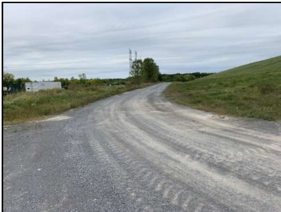
Photo 40: View facing north of potholes present on the southwest access road, northwest of the base of the landfill mound access road.
