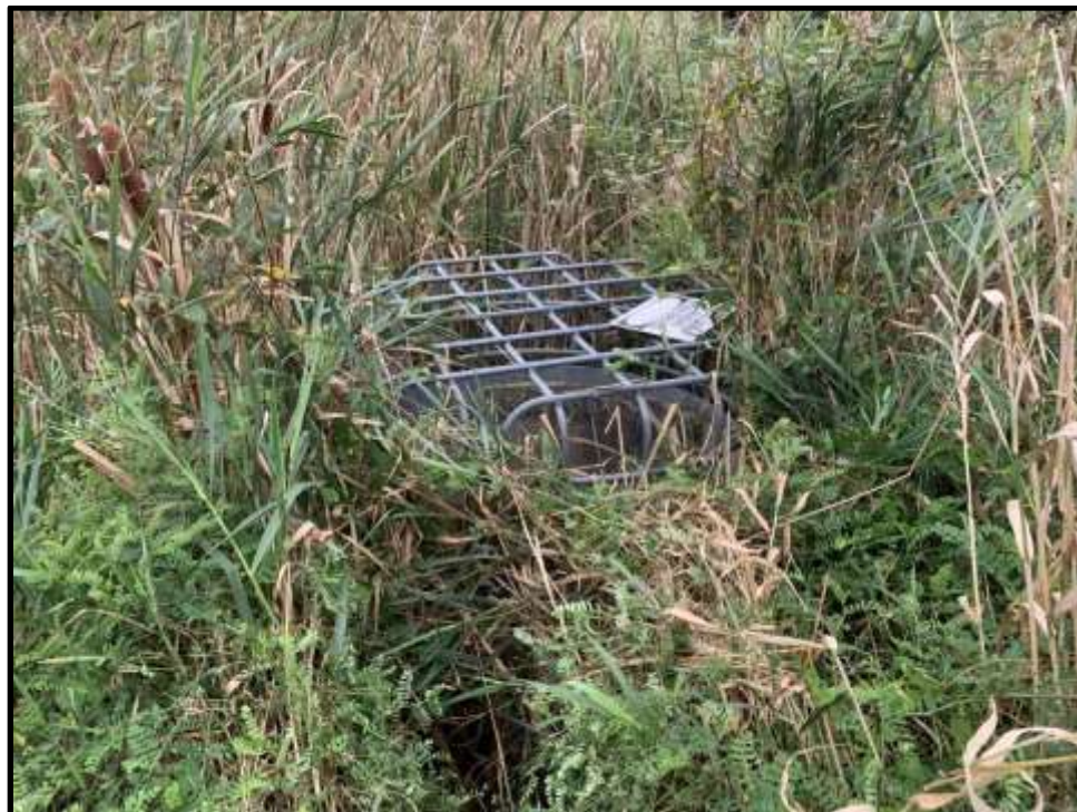
Photo 20: View facing south of the drop inlet pipe spillway structure at Stormwater Pond 2. Vegetation is obscuring access.
