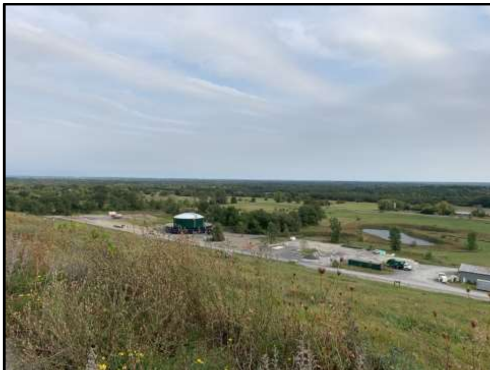
Photo 44: View facing southeast of progress on the leachate storage system construction project
