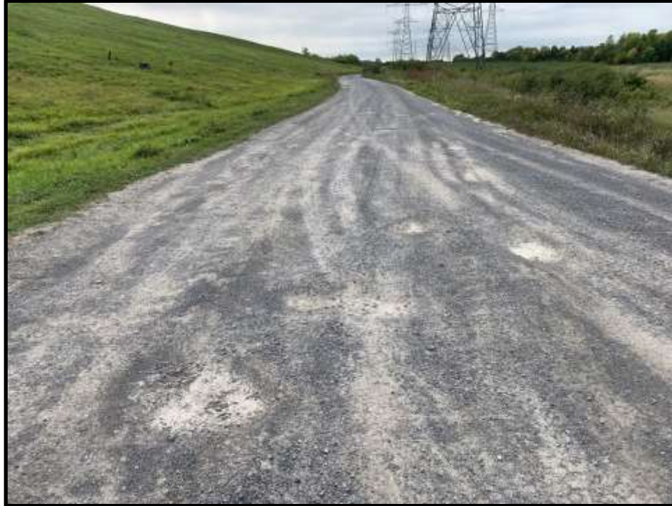
Photo 39: View facing west of potholes present on the north central access road, west of the north chamber.
