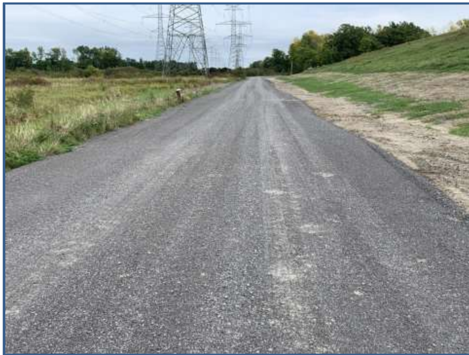
Photo 36: View facing east of granular material placed on the northeast access road, as part of the leachate forcemain installation restoration activities.
