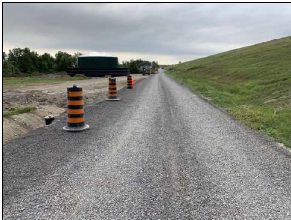
Photo 38: View facing south of granular material placed on the southeast access road as part of leachate forcemain installation restoration activities.
