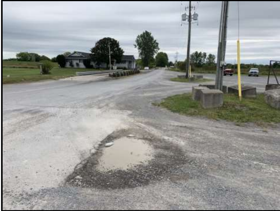
Photo 41: View facing south of a pothole present on the west side of the tee intersection at the maintenance building.
