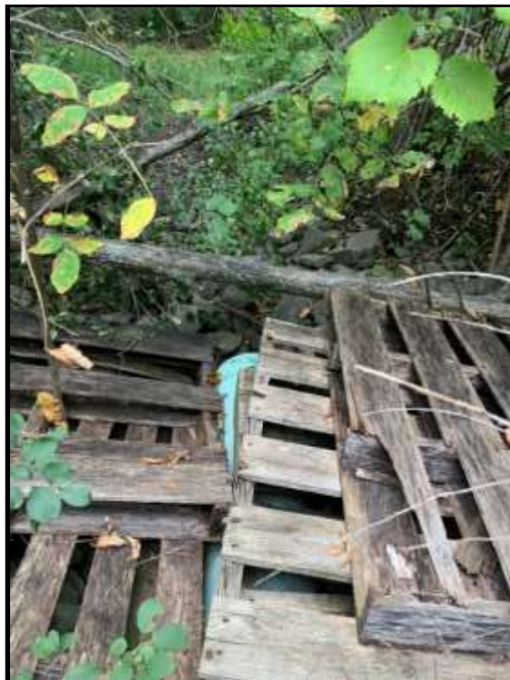
Photo 22: View of the outlet pipe from Stormwater Pond 2. Wooden pallets allow for access during high flows but are not considered to be a stable walking surface. No evidence of silt exiting the site was observed.
