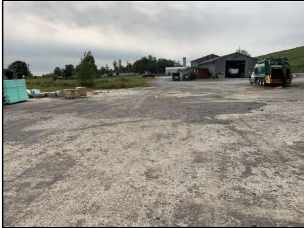
Photo 43: View facing west of the southwest side of the former contaminated soil pad. Potholes are present and the area has exhibited wear.
