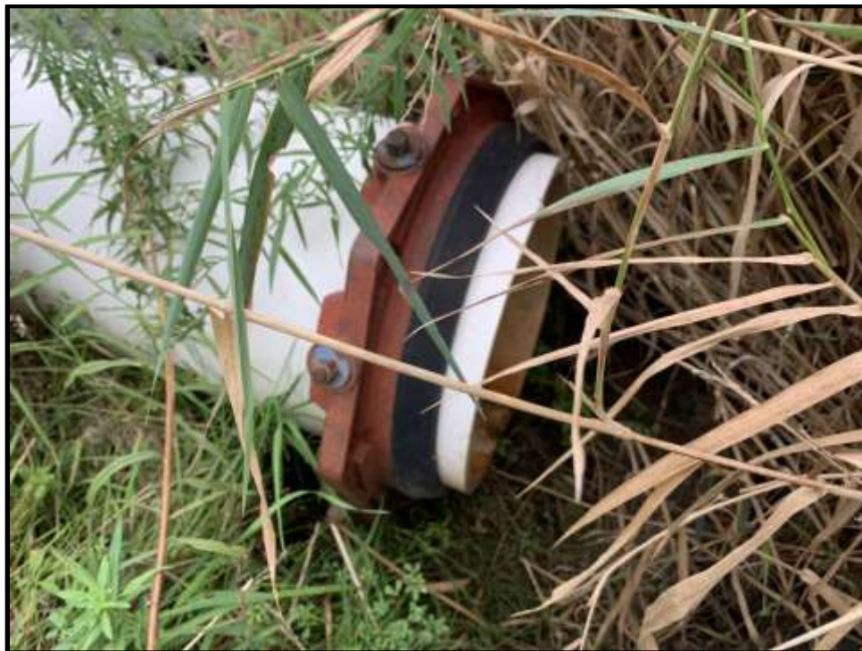
Photo 12: View of the outlet pipe at the west end of Stormwater Pond 3. The outlet is becoming obscured by vegetation.
