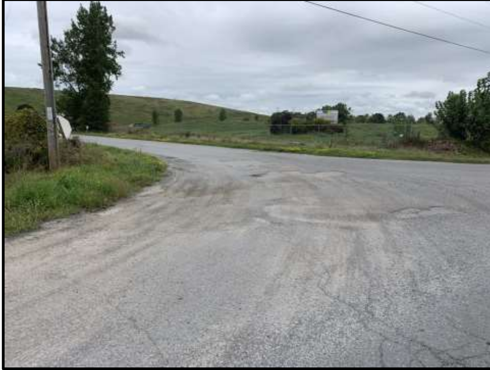
Photo 1: View facing north of the pavement at the site entrance off Beechwood Road. Potholes have been filled with granular material.
