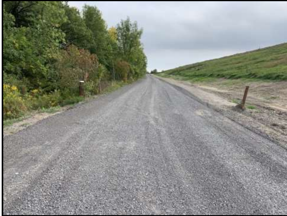
Photo 37: View facing south of granular material placed on the east access road as part of leachate forcemain installation restoration activities.
